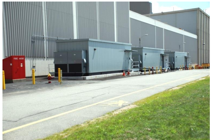
Figure 7. VFDs In Operation at Millstone
